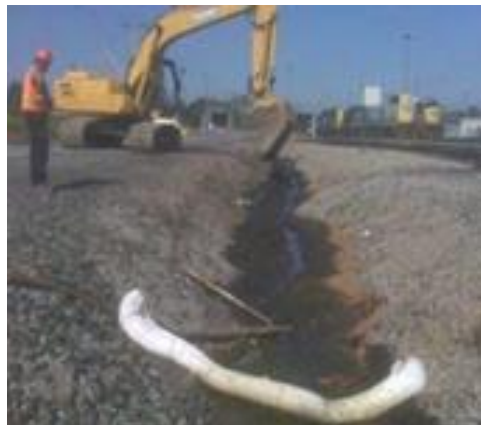
Petroleum Impacted Drainage Ditch
