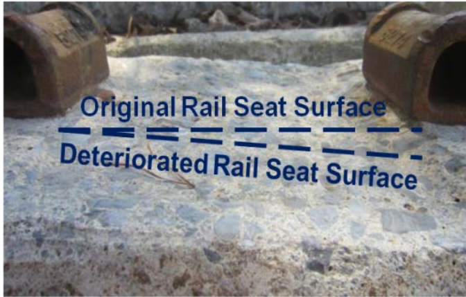
FIGURE 1. EXAMPLE OF RAIL SEAT DETERIORATION
