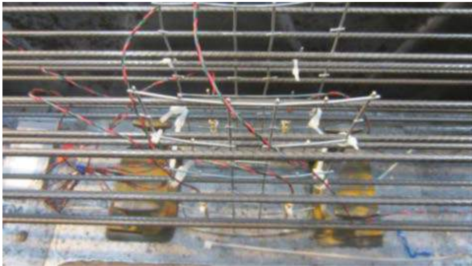
Figure 23. Mesh to Hold Embedded Crosstie Strain Gauges Prior to Concrete Being Poured
