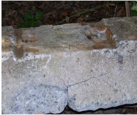
Rail seat positive flexural cracking
