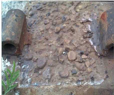
Rail seat deterioration
