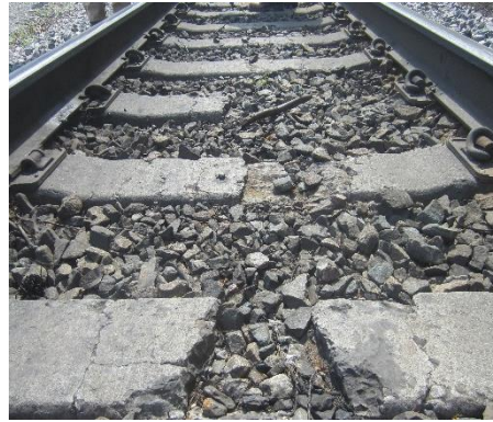
Center negative flexural cracking
