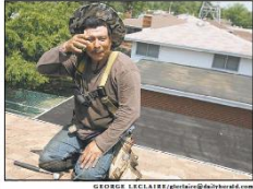
AMANDO GARCIA WITH LINDBERGH ROOFING WIPES HIS FOREHEAD WHILE WORKING ON A ROOF IN DEER PARK ON THURSDAY. GARCIA SAID IT WAS ABOVE 100 DEGREE ON THE ROOF.
