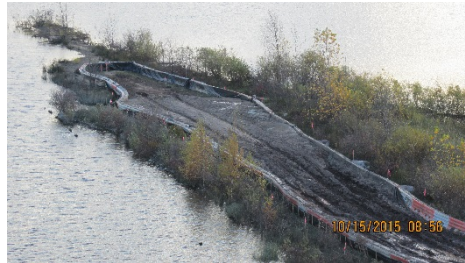
Excess slurry on spit
