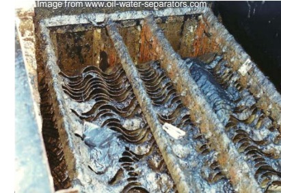
Clogged Coalescing Media
