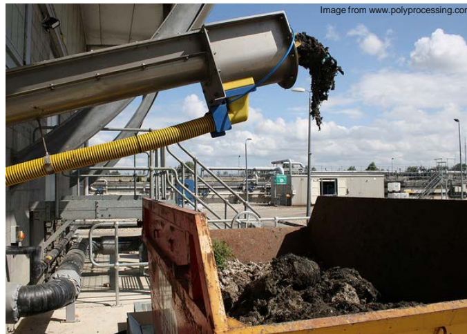
Dewatered solids are collected to be hauled for offsite disposal
