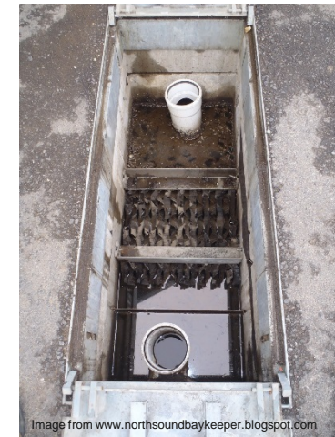
Partially Drained Oil/Water Separator
