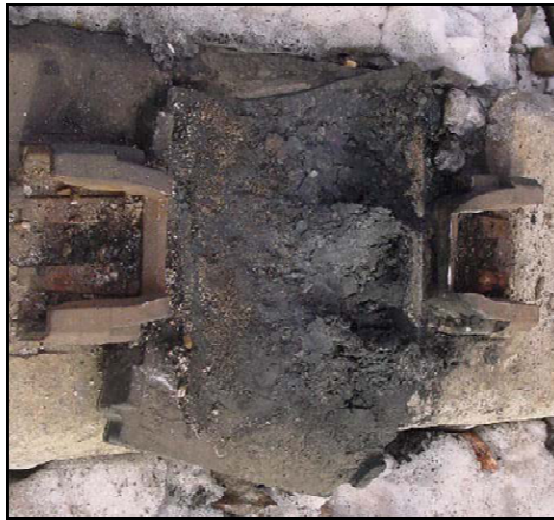
Figure 2.6 Example of tie pad wear (Humphreys 2007)
