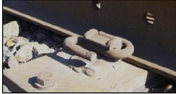
Figure 2.5 Severe example of loss of clip toe load (sprung clip)
