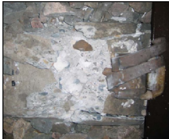
Figure 2.4 Severe example of a shattered concrete shoulder and a yielded clip, caused by a derailment impact (Humphreys 2007)
