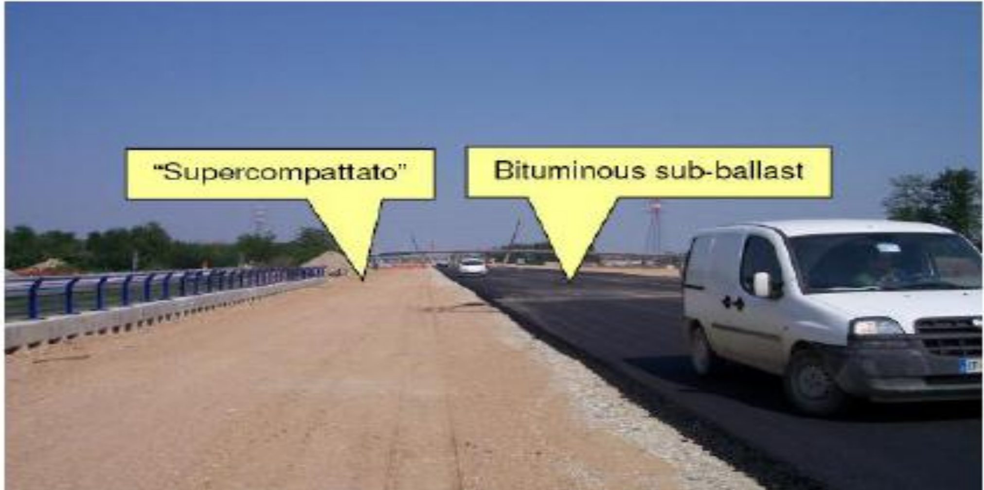
Italian Trackbed Construction – Improved Subgrade on left, prior to addition of Granular and Asphalt Subballasts on right
