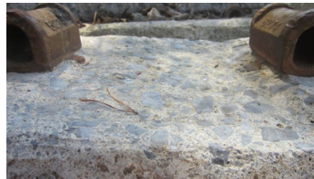
Rail seat deterioration
