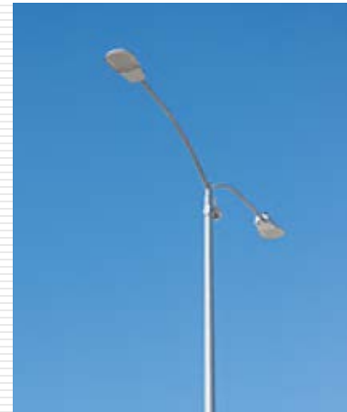
40' Entrance Road Fixture
