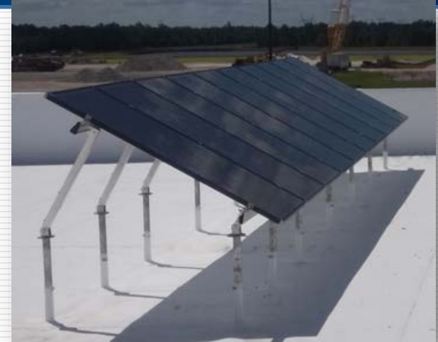
Solar panels on the roof of a Winter Haven facility building
