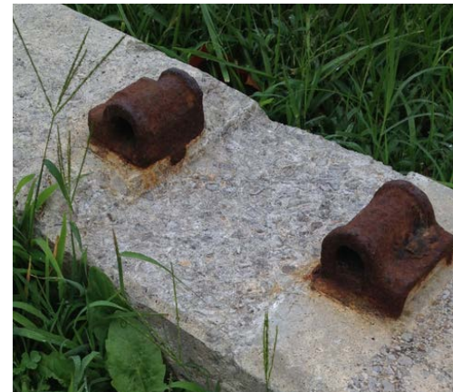
Rail Seat Deterioration
