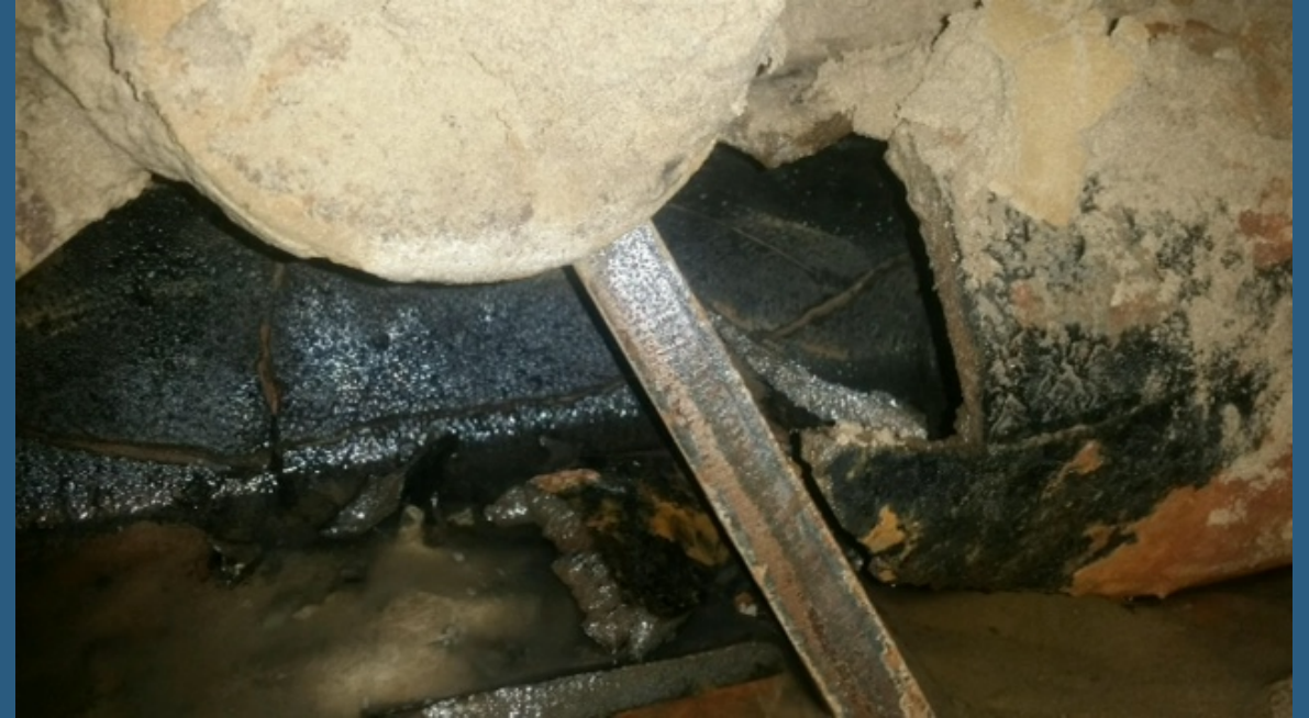
Abandoned water line (unmarked) – hit during jack and bore (view from inside of steel casing)
