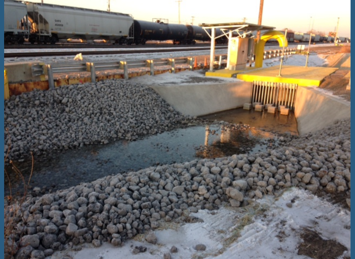
Completed lift station with rip-rap lined channel inlet, trash grate, and electrical control panels
