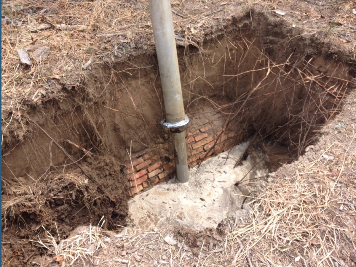
Brick sewer side view during nozzle retrieval (note groundwater and mortar conditions)
