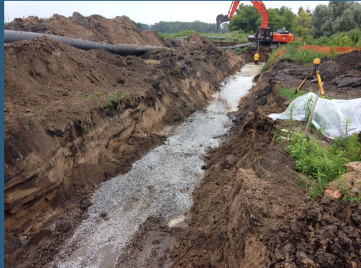
Removal of brick sewer top and sides, and placing stone bedding (fly ash placed on Visqueen and covered)
