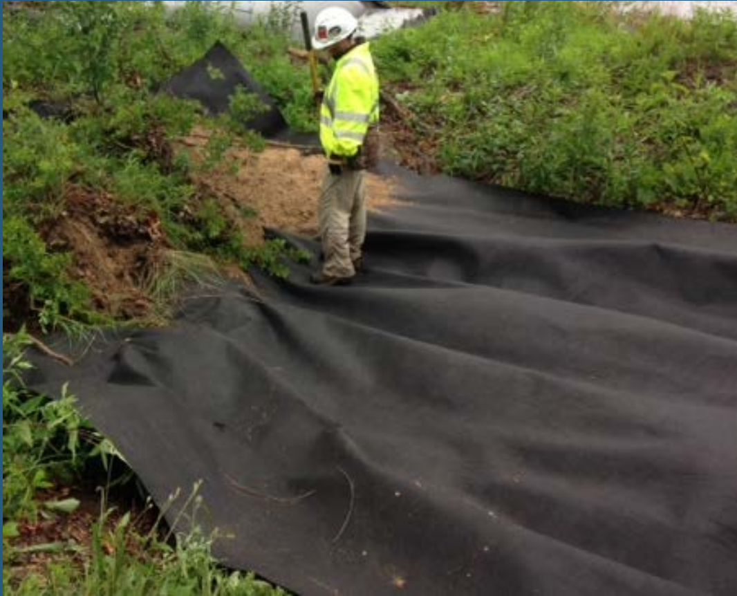
Some plants were staged on geotextile to allow for trenching to be completed and backfilled
