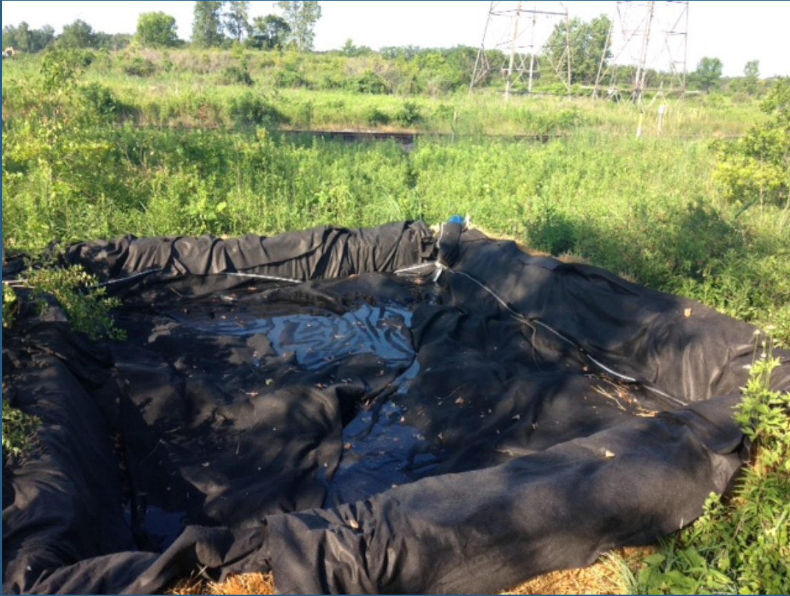
Dewatering filter basin: geotextile filter bag set inside straw bale basin lined with additional geotextile
