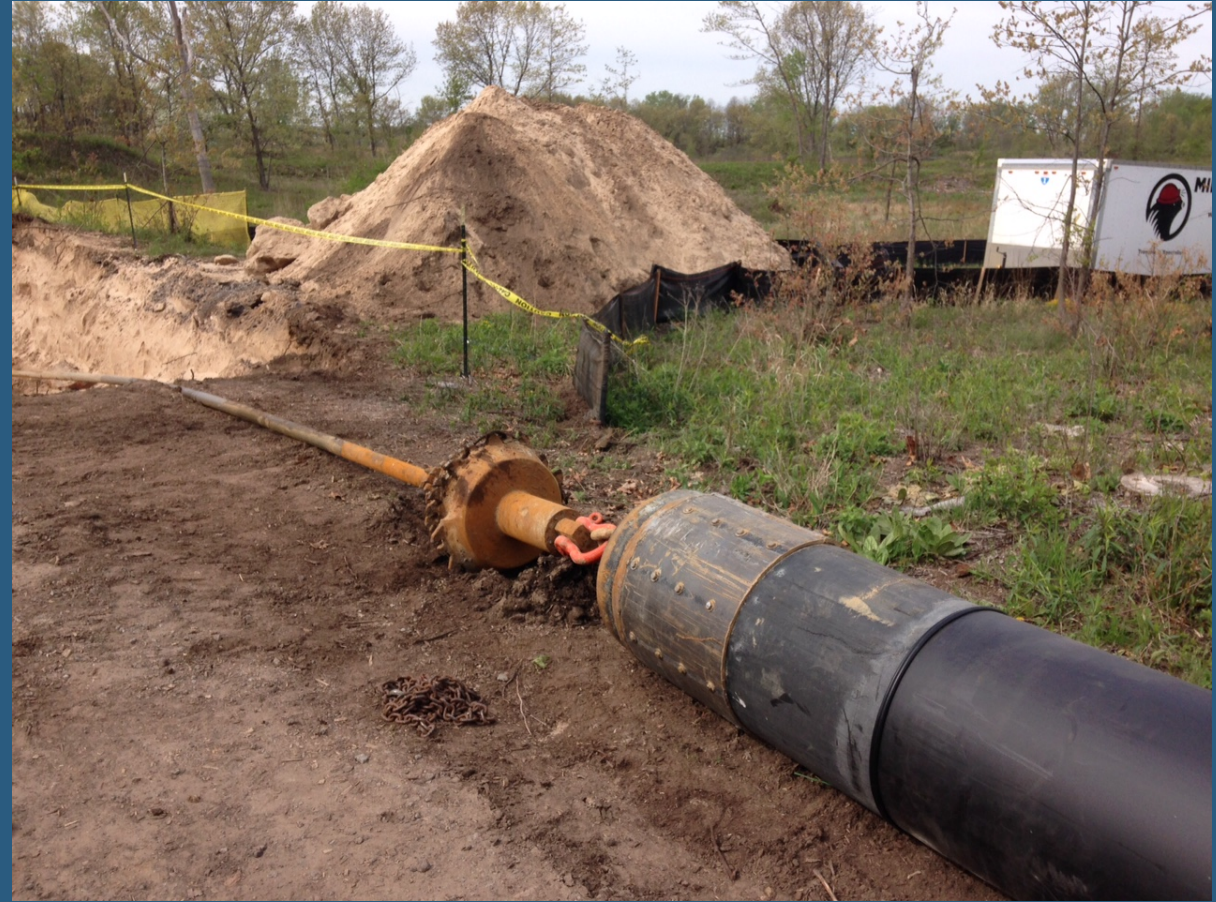
Reaming head connected to liner pipe, ready to pull into entry pit
