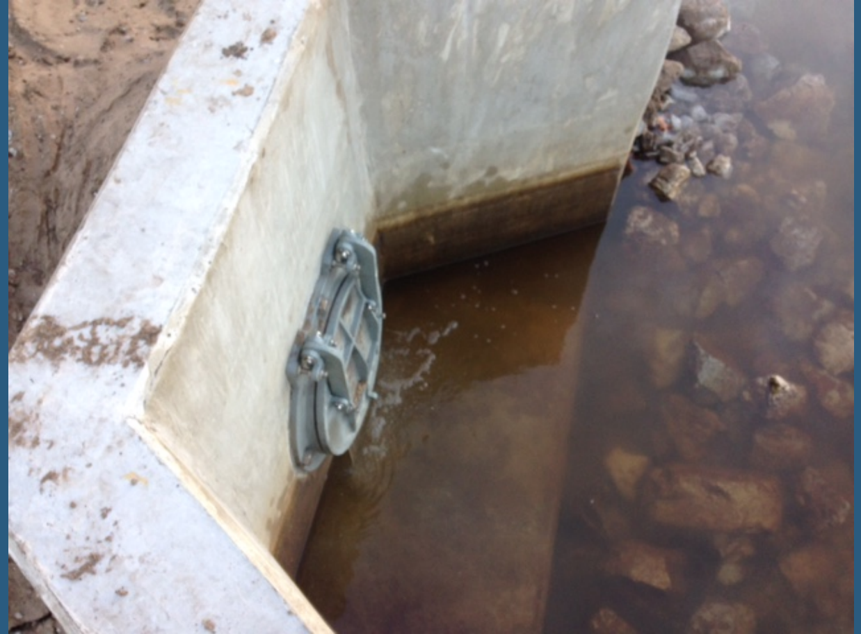
First discharge at new outfall to Grand Calumet River
