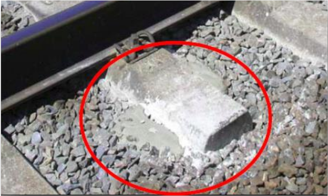
Deterioration of ties and ballast
