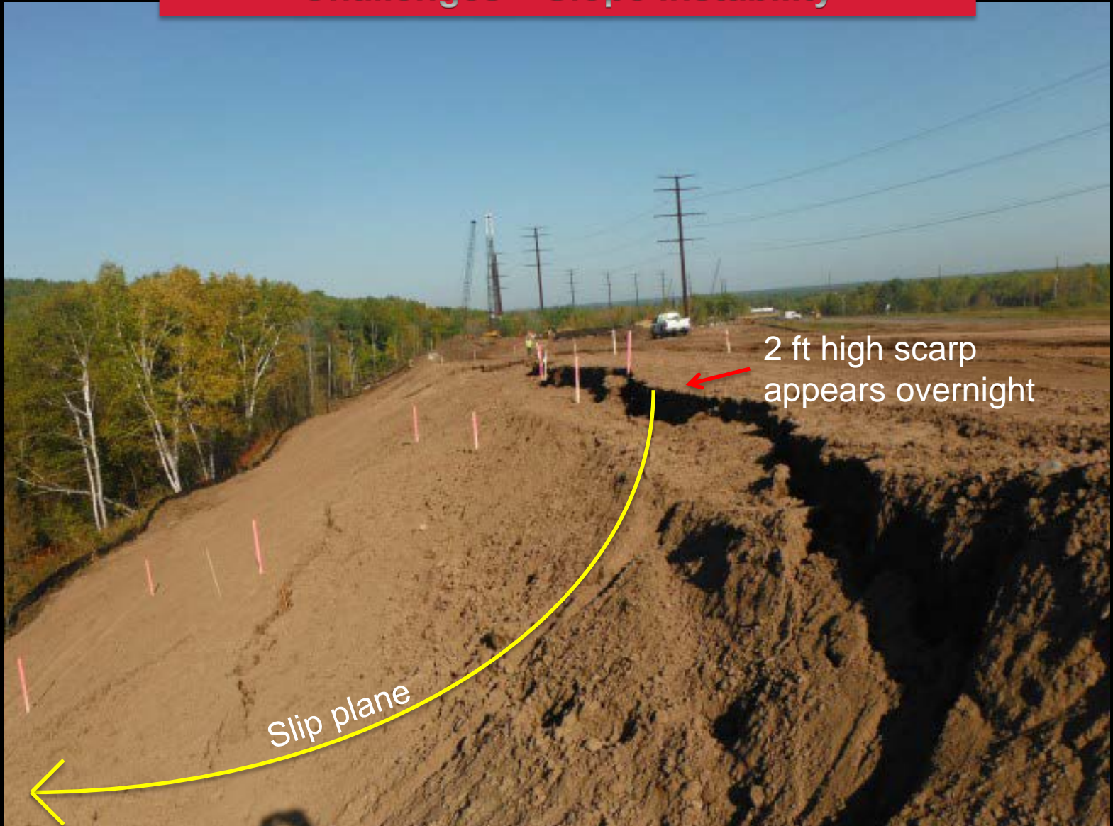
Slope failure – 300 ft long, 30 ft high
