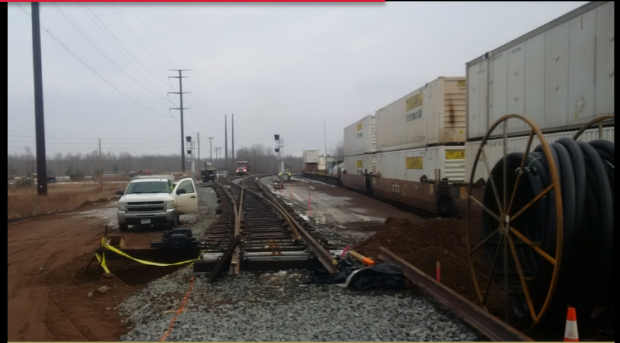
New power switches
