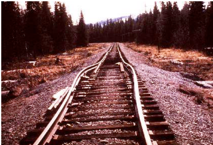
Figure 2.3. Buckled rails due to lateral movement of the embankment over a crushed culvert (Abston and McGregor, 1995)
