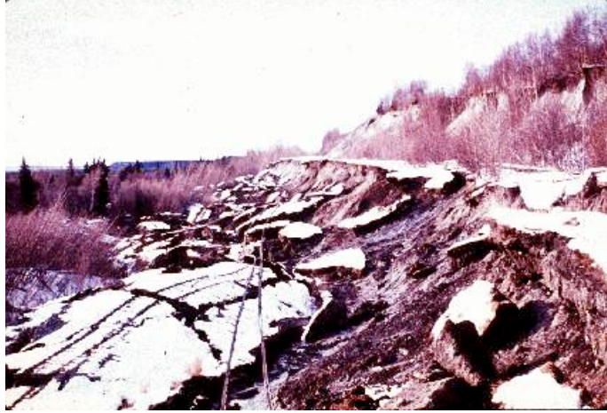
Figure 2.2. Earthquake-triggered landslide on the Alaska Railroad mainline near Potter Hill (Abston and McGregor, 1995)
