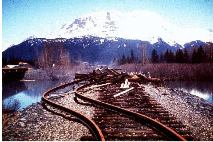
Figure 2.4. Rails that buckled due to channel movement of the riverbanks during the 1964 Alaska earthquake (Abston and McGregor, 1995)
