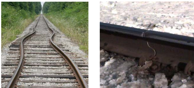
Figure 1.1 Compression and Tension Failures in Rail (photo by D. Uzarski, 2005)
