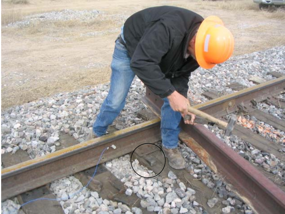
Figure 9.10 Steel Wedges Between Tie Plates and Timber Ties
