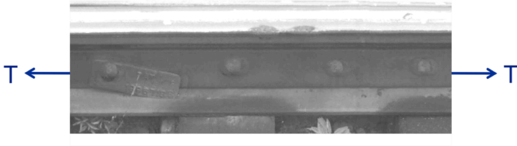
A: Original Image Switch Point Bolts.
