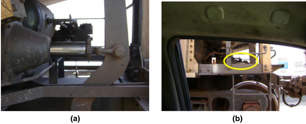
Figure 3.9 Extended Brake Piston (a) and View of Piston from Inspection Vehicle (b)
