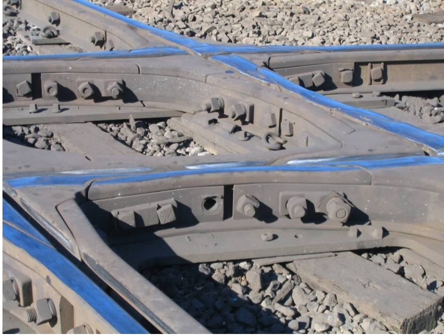
Figure 7.3: Crossing Diamond with Missing Bolts and Fasteners on FRA Class 4 Track
