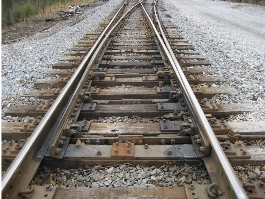
Figure 2.4: View of a Turnout Showing the Switch, with the Points Aligned for the Straight (Normal) Route
