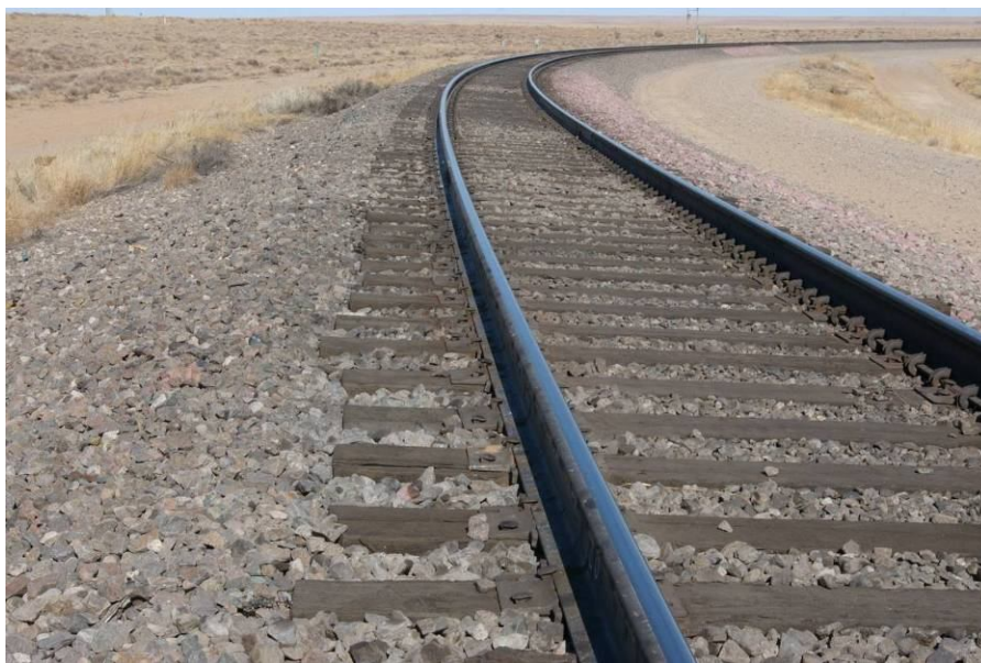
Figure 6.2: Image from Ballast View Recorded at the Transportation Technology Center's (TTC) Facility for Accelerated Service Testing (FAST)
