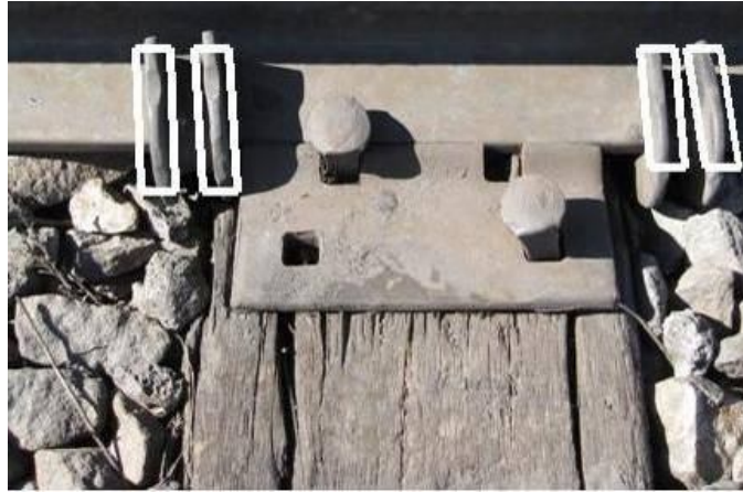
Figure 8.6: Anchor Detection Results Showing the Detection of Channel Anchors
