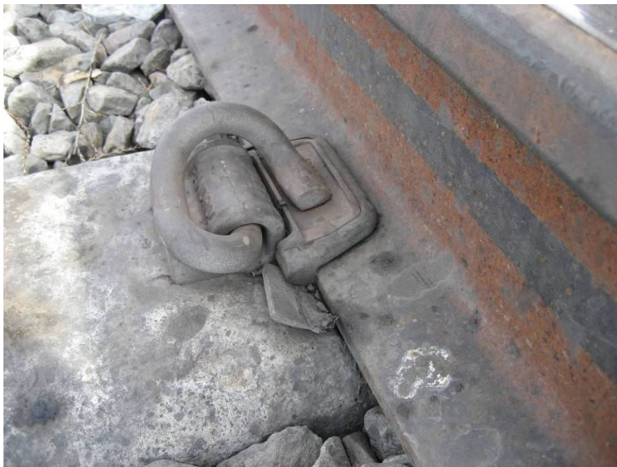
Figure 9.1: Image of Fastening System with Tie Pad Wear and Possible Rail Seat Abrasion
