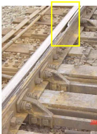
Figure 3.8: Example of Switch Point Chipping
