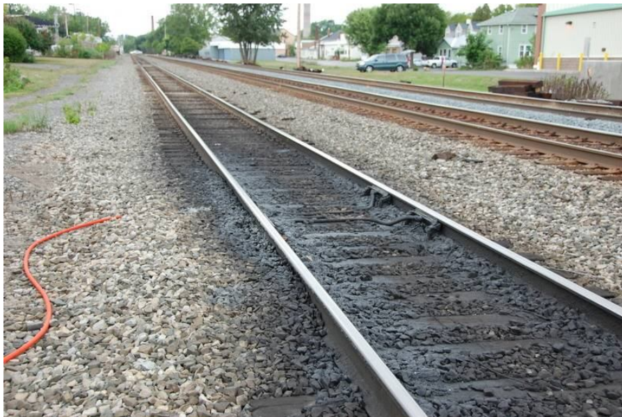
Figure 9.2: Image of Operative Rail Lubricators Showing Grease on and Near the Tracks
