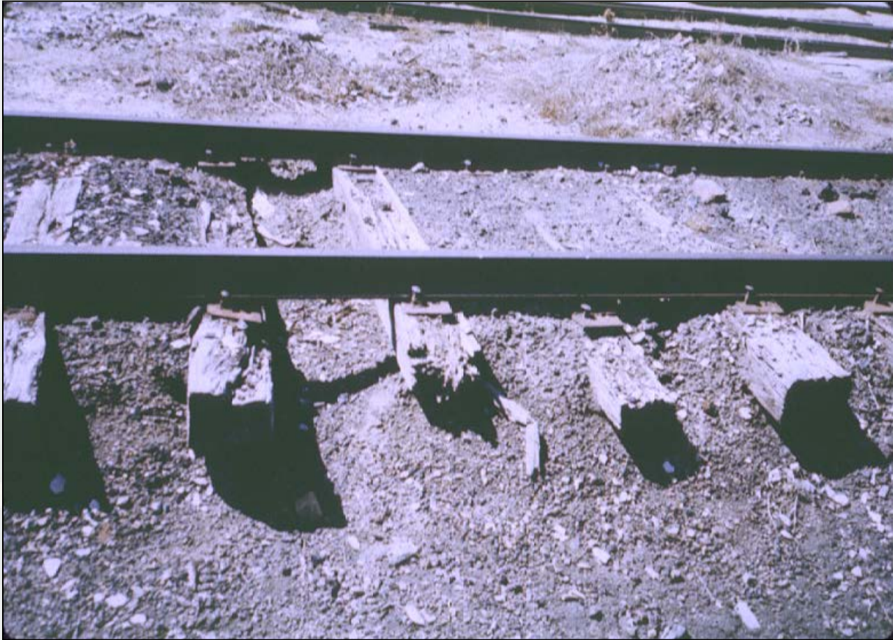
Badly Deteriorated Wood Cross-ties
