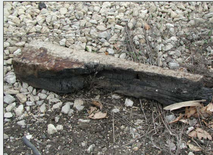
Burnt wood tie
