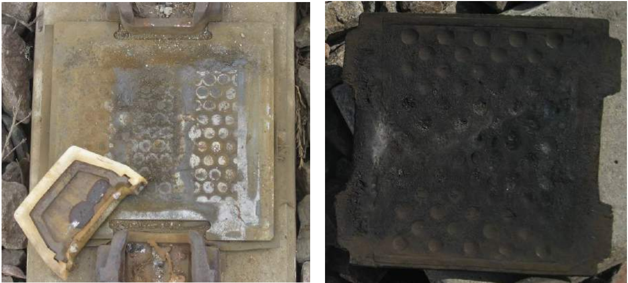
Figure 2.4 Worn dimples and grooves on rail pad assemblies
