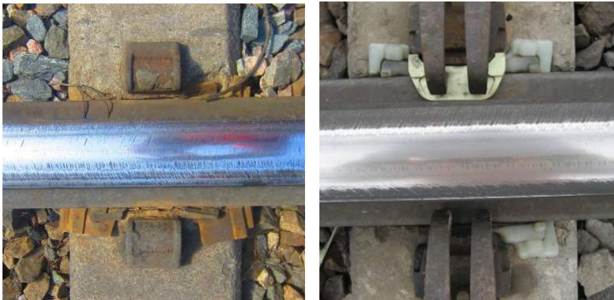
Figure 2.3 Crushed rail pad assemblies
