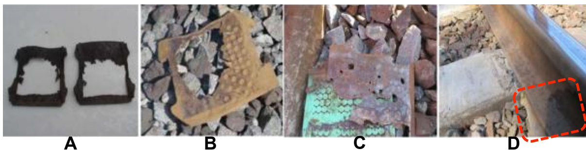
Figure 1 - Failure modes associated with rail pad assemblies [10]
