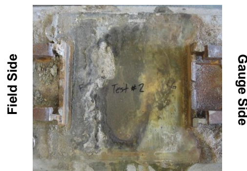
Figure 3: Worn rail seat surface treatment on the field side after 3 million cycles
