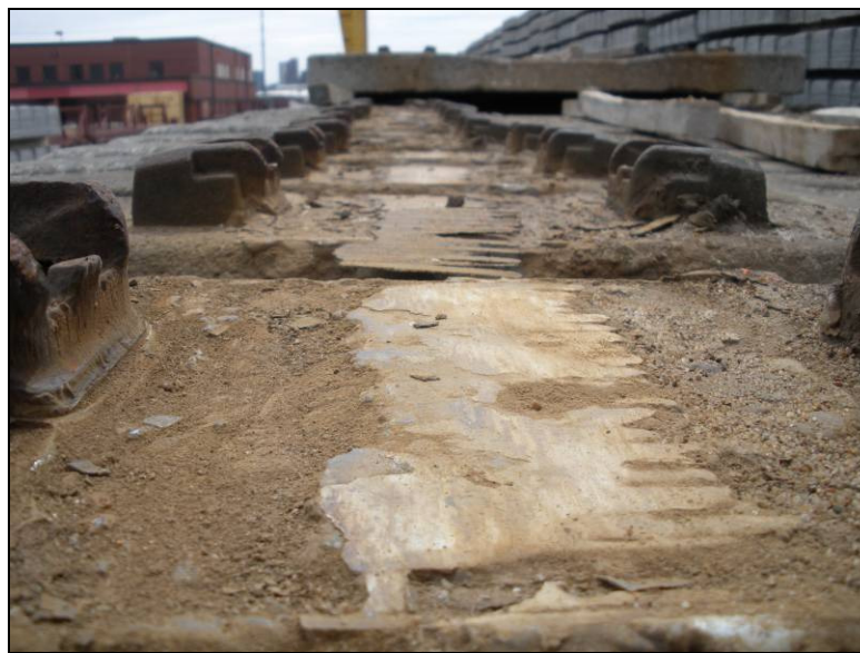
FIGURE 2. Service Example of Rail Seat Deterioration
