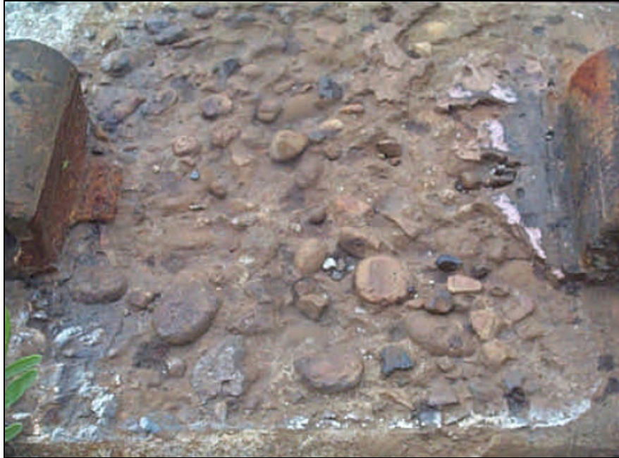
FIGURE 3. Service Example of Rail Seat Deterioration
