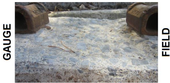
Figure 1: Typical Rail Seat Deterioration (RSD) Wear Pattern
