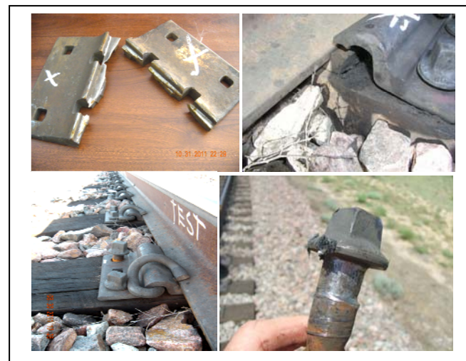
Figure 3. Clockwise from top left corner – Broken AREMA 14-inch Tie Plates, Broken Rolled Tie Plate, Screw Spikes with High Neck Wear, and Broken Screw Spikes
