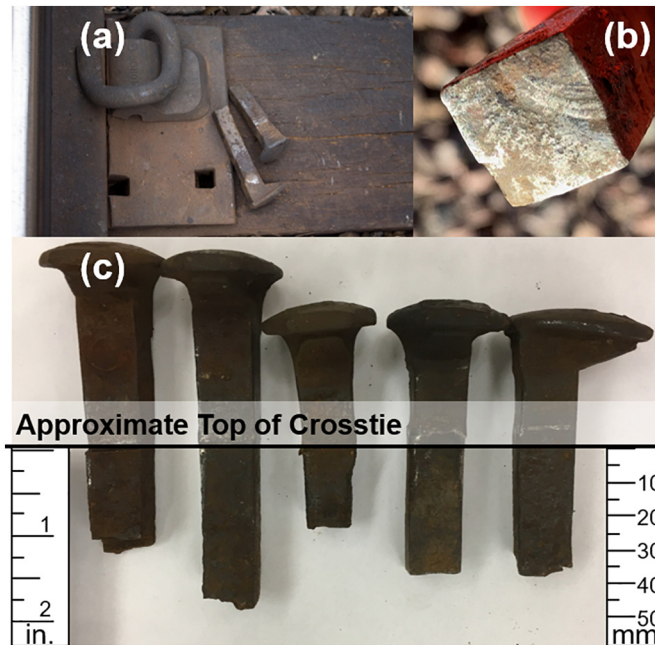
Fig. 1. (a) A premium fastening system found to have two broken spikes. Broken spikes were found and removed from the crosstie during a walking inspection. (b) Example fracture surface of a broken spike. (c) Examples of broken spikes with varying depths of failure location found during walking inspections. Measurements in inches.
