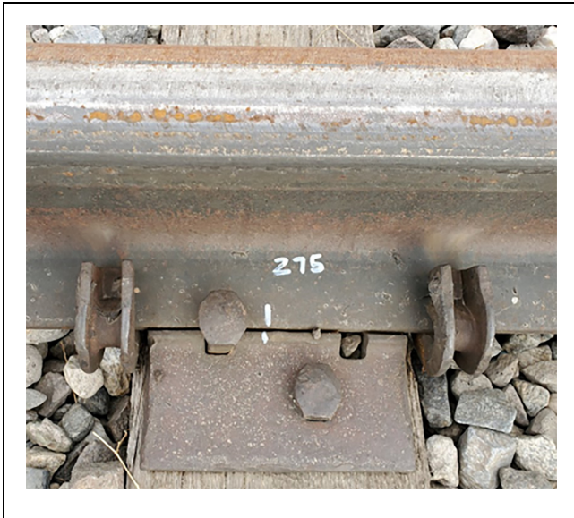
Figure 4. Example of a match-mark placed on the rail and plate 83.8 m (275 ft) away from the cut.
