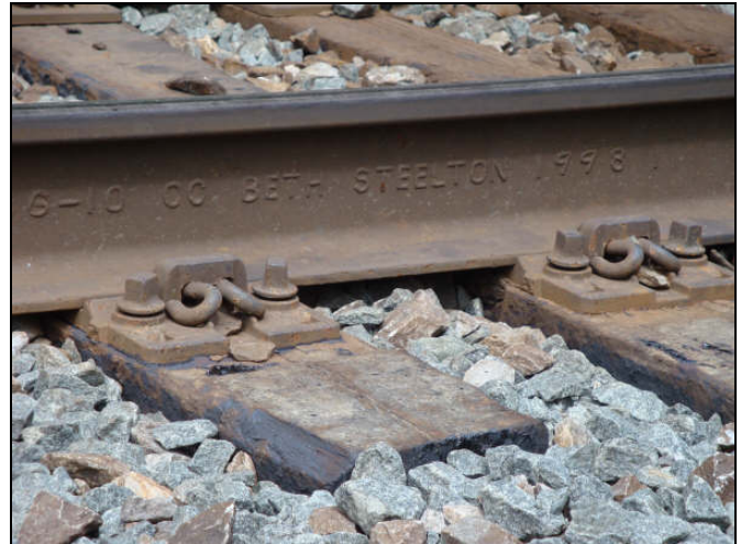
Figure 7. Gap between the Screw Spike Head and Tie Plate after the Tie-Bottom Cleats seated into the Wood Fibers
