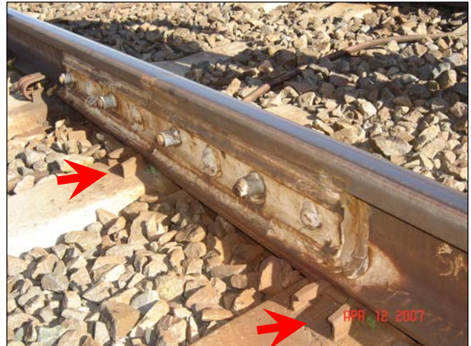
Figure 2. Example of Missing Fasteners in Revenue Service
