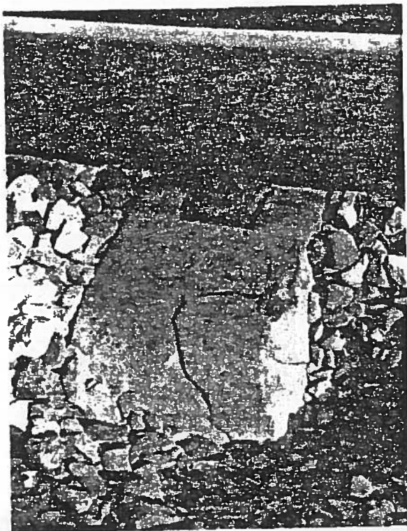
PLATE 34. TIE DAMAGE ATTRIBUTABLE TO INSUFFICIENT BALLAST
