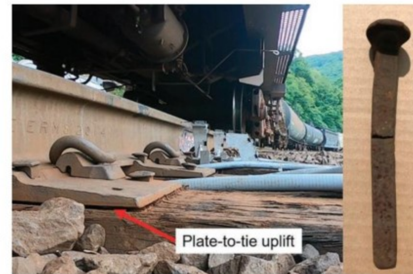
Figure 2. Examples of plate-to-tie uplift and of damaged spike.
