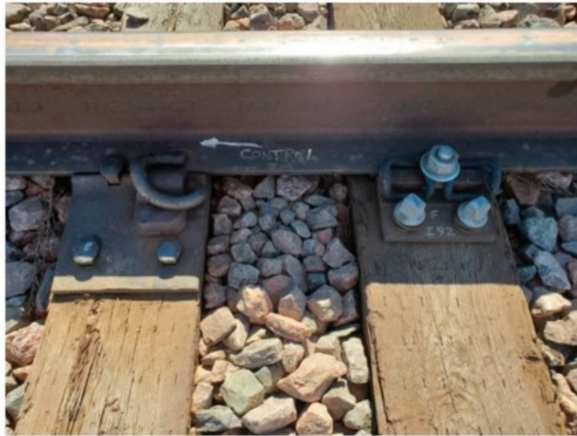
Figure 7. Transition between control zone (left) and test zone (right) at TTC FAST, 2019-2020.
