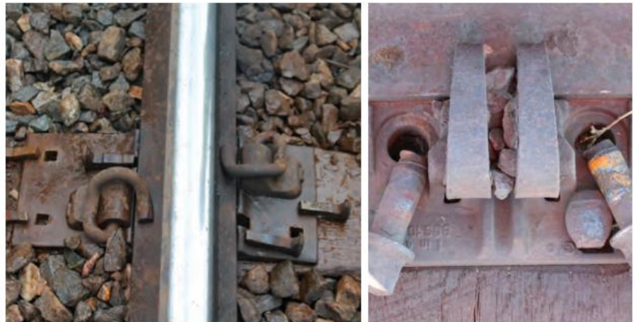
Figure 1. Premium elastic fastener with five broken spikes and broken lag screws in McKay fastening system.
