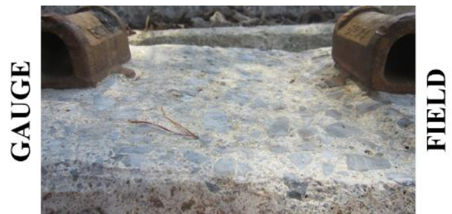
Figure 1. Typical Rail Seat Deterioration (RSD) Wear Pattern
