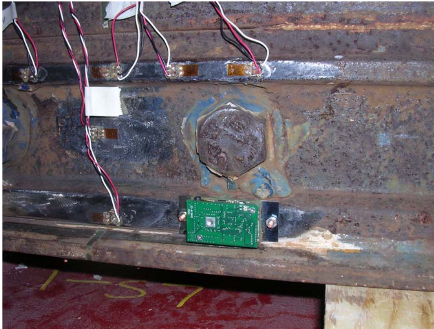
FIGURE 28 Sensor installed on an insulated joint
